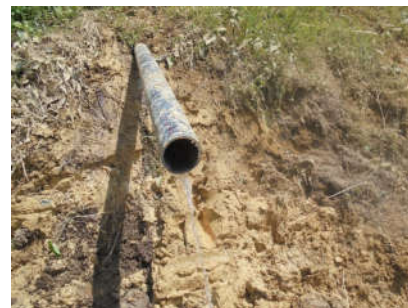
Water discharge from horizontal gravity drains
