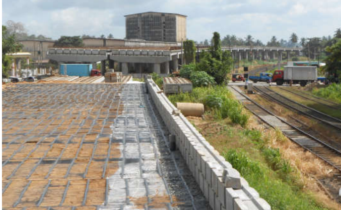
Reinforced Earth Retaining wall to provide approach to Viaduct at Hunupitiya -CKE
