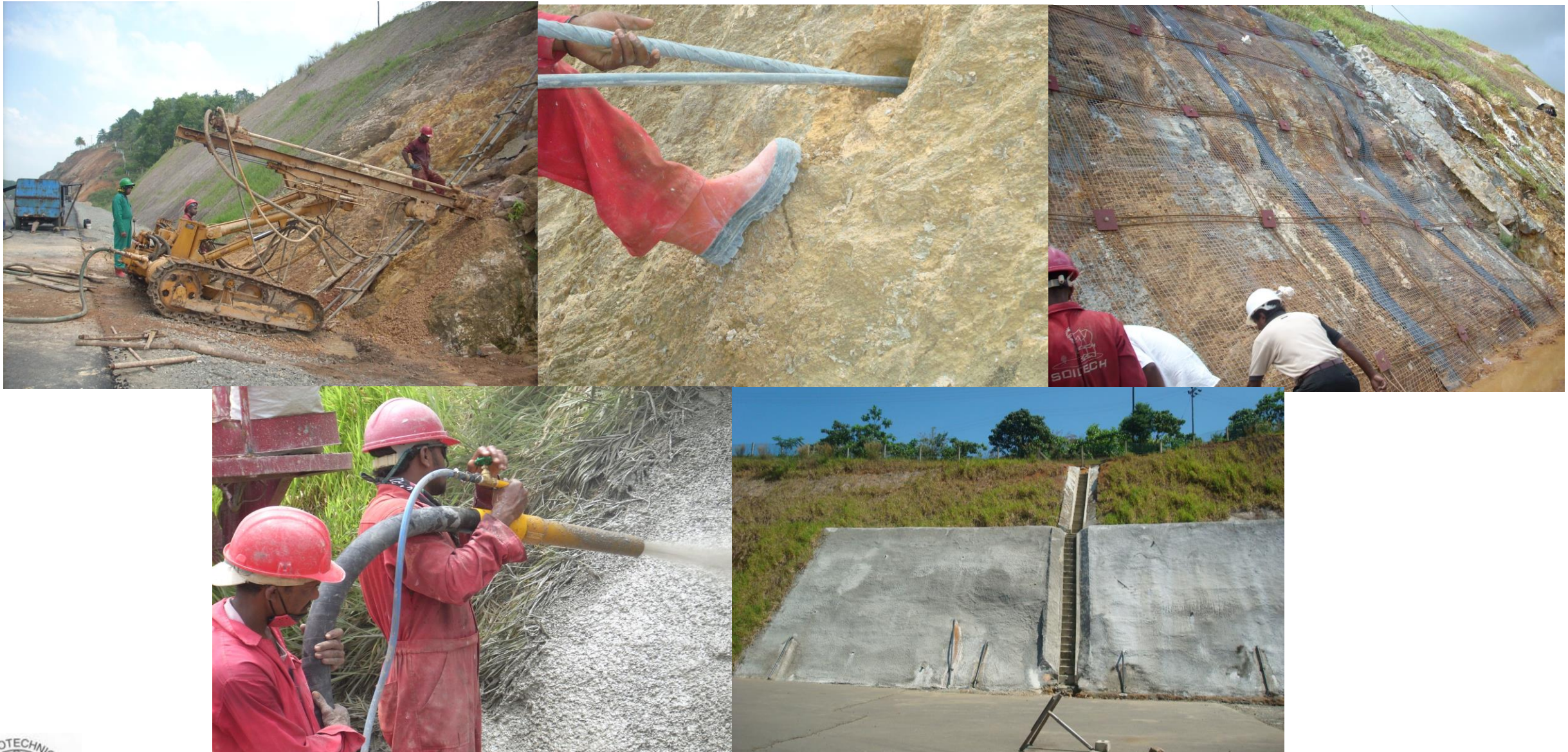
Drilling the hole, installing the nail and grouting, placement of reinforcement and shotcreting
