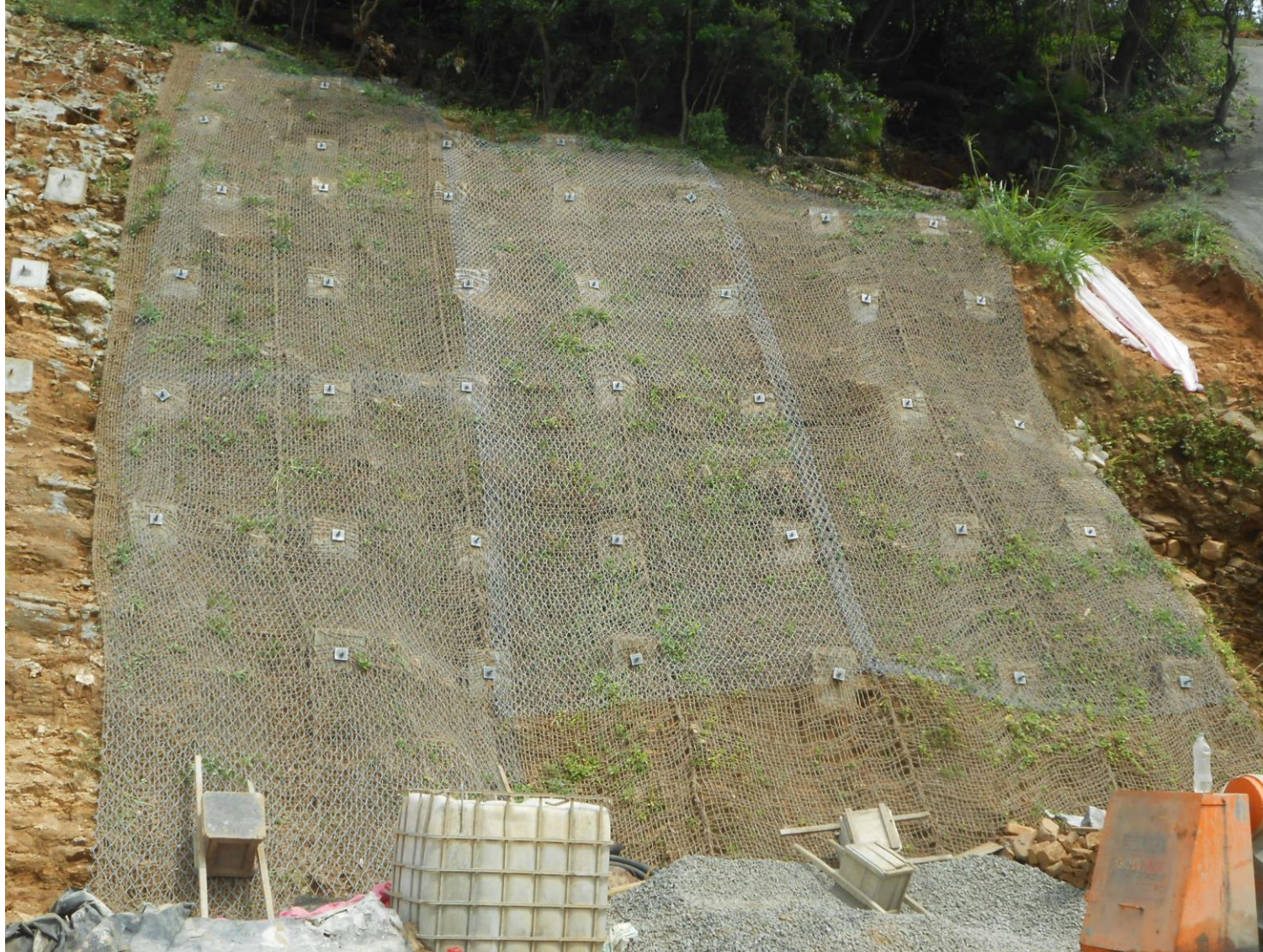
Protective net and coir mat introduced to provide surface cover by hydro seeding Location 10 Kandy Mahiyangana Road
