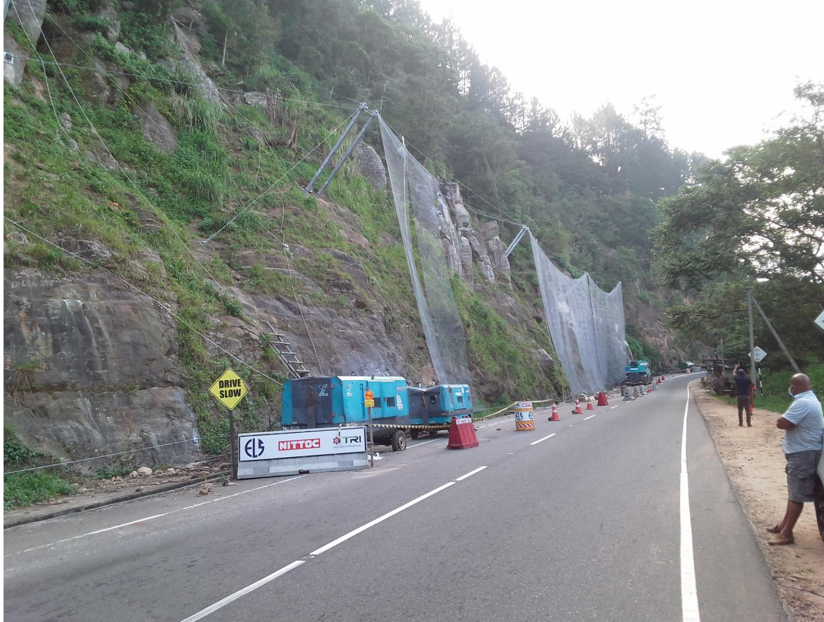
Curtain Netting to retain falling rock pieces Kandy - Mahiyangana Road
