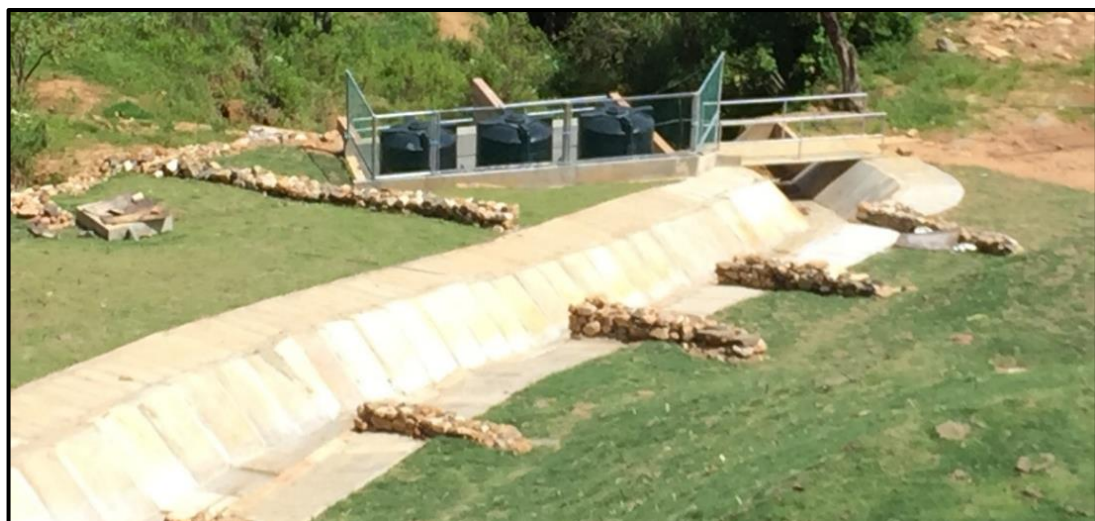
Figure 4.6: Outlet of Surface drainage system (A2 in figure 4.3)
