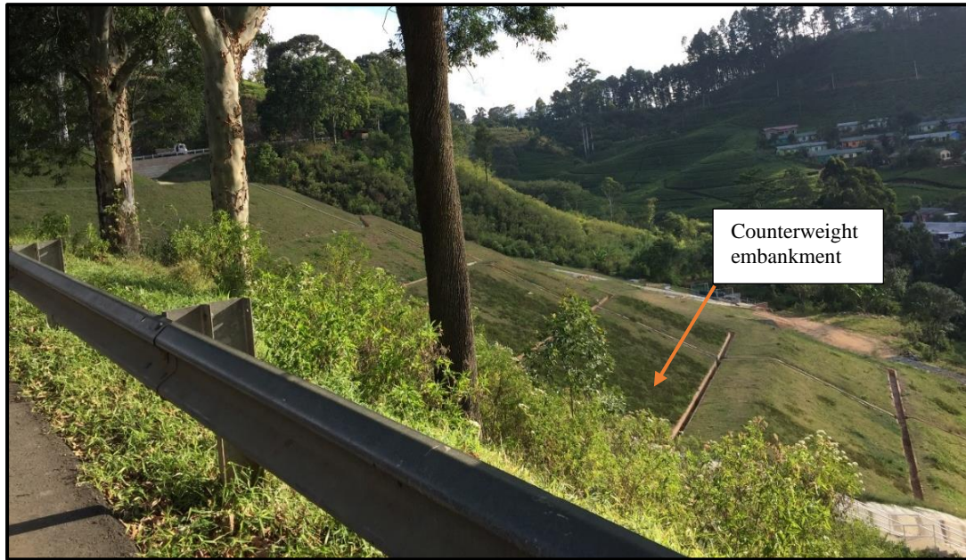
Figure 4.9: Counterweight embankment work at the landslide toe area (B1, B2 in figure 4.3)
