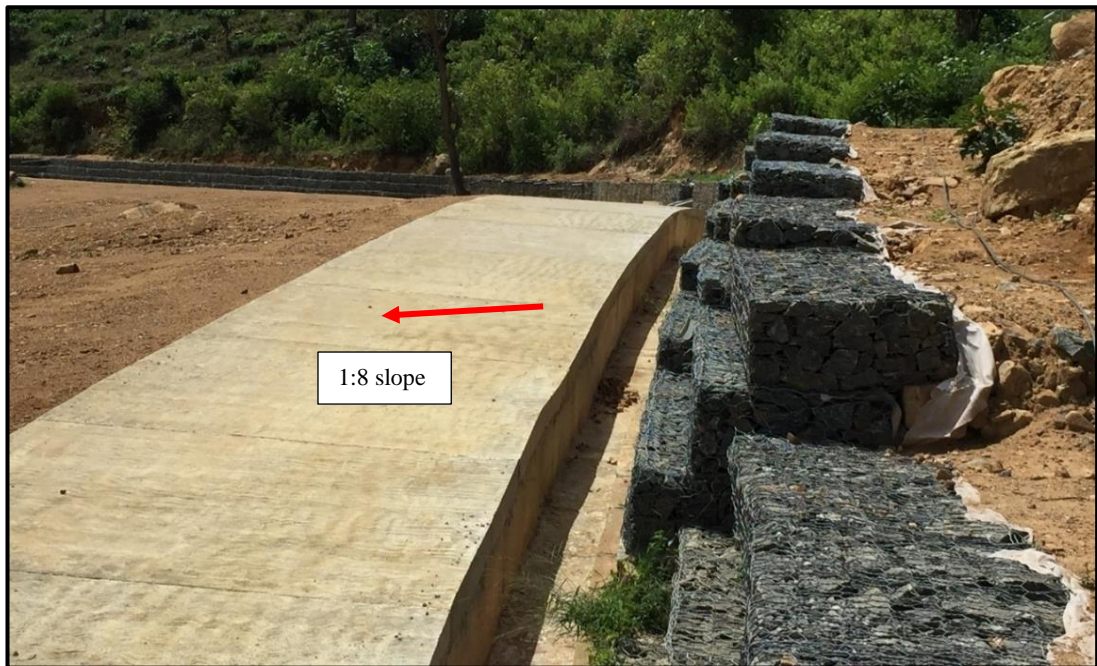
Figure 4.7: Earth removal and slope protection at the Landslide upper area (D4, D5, E4, E5 in figure 4.3)
