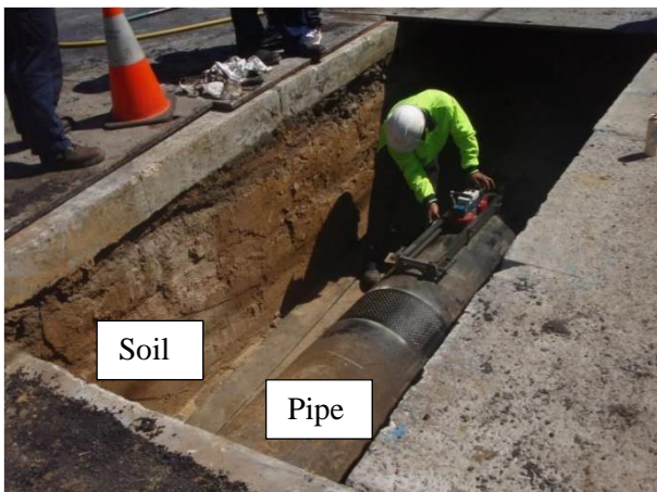
Fig. 1 Location of the soil sampled after excavation to expose a large water pipe.
