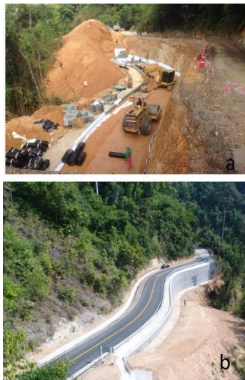
Fig. 6 The studied geosynthetic-reinforced soil wall; a) during construction; b) completed wall (viewed from a different angle)
