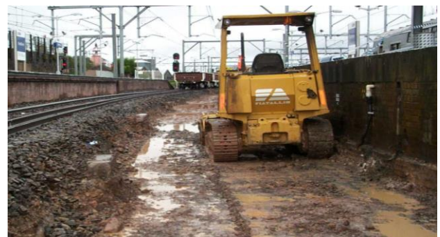
Fig. 1 A railway site which is prone to mud pumping near Wollongong in New South Wales, Australia
