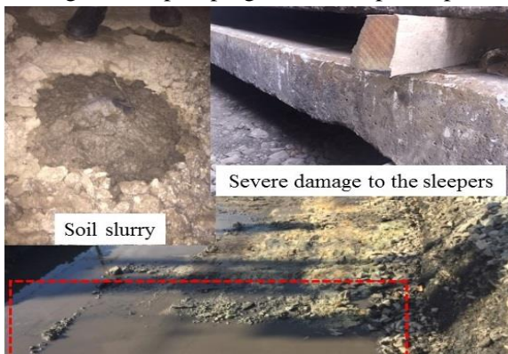
Fig. 1: Perched water table on the subgrade surface at a problematic site near Wollongong City, Australia.
