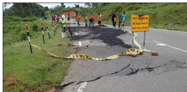
Fig.1. Road cracks appeared during rainy period (Photo taken on 26-12-2014)
