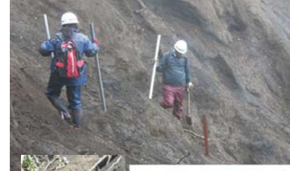
Monitoring & early warning for secondary failures
