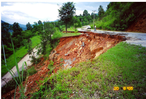
Fig. 2 Failure of the back and filled slope
