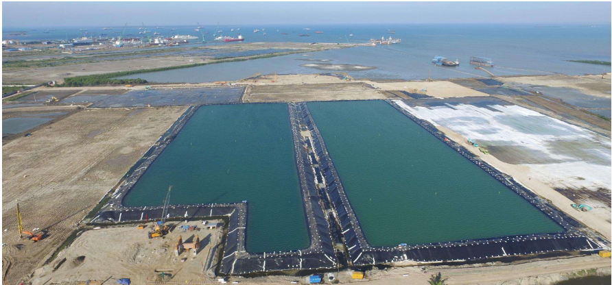
After VCM + Water Surcharge improvement, the ground settle 1.4~1.5 m and the unconfined shear strength S_u increase 18~25 kpa
