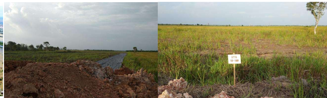
Water table will be decreased to 1m below ground during dry season.
