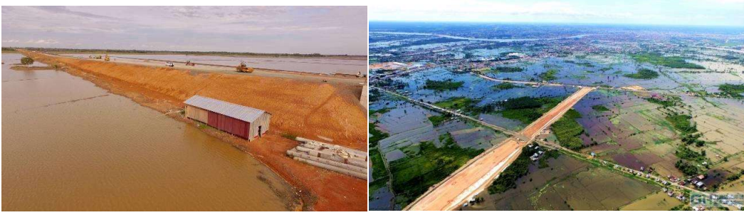
Water table will be increased to 1.5~2m above ground during rainy season.
