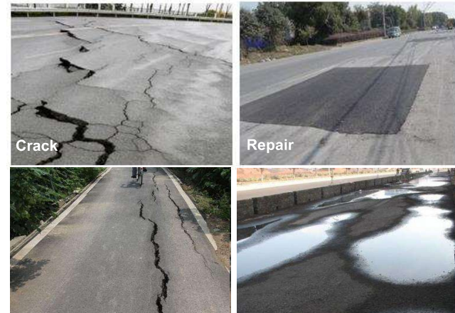
Problem of Settlement for Road
