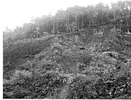
View of the Right Flank of the Landslide from the Toe
