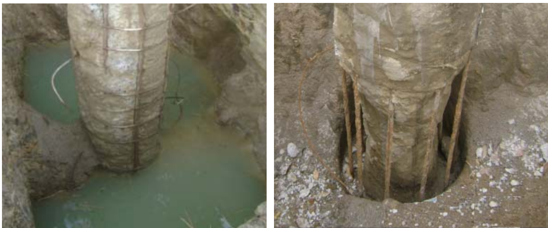
Figure 1 – Defective piles exposed by excavation.
