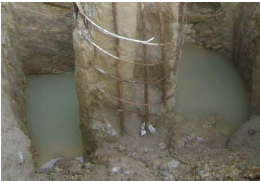
Figure 8 A defective pile exposed by excavation.
