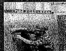
3. Hold at the left hand side by a strip nailed into the wall, the rest of the area is secured by plugs. The overlap is secured by lashing.
