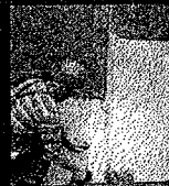
5. Additional lashing may be required to secure the overlaps and the covering to the pipe at the bottom of the well.
