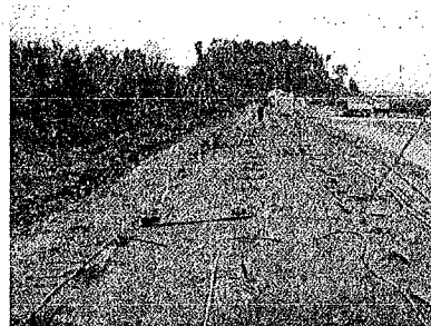
Figure 7: View of EVD with cables attached
