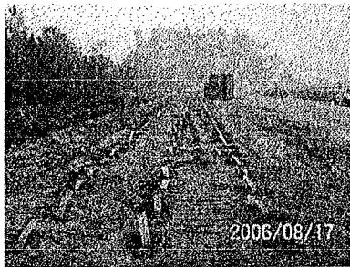
Figure 6: View of EVD installed
