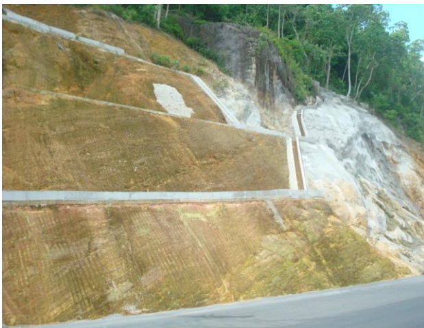
Figure 6 - Use of Sealed drains over the berms and cascade drains in the STDP
