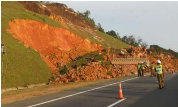
Figure 5: Initial Crack & downward movement of soil
