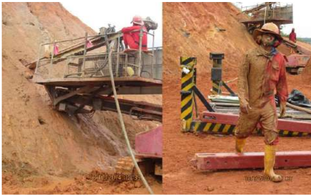
Figure 2: Water oozing out of relict joints during drilling and covering the workmen in mud
