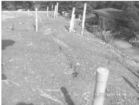
Figure 14. Figure showing tilt of inclinometer at the top of RSS facing.
