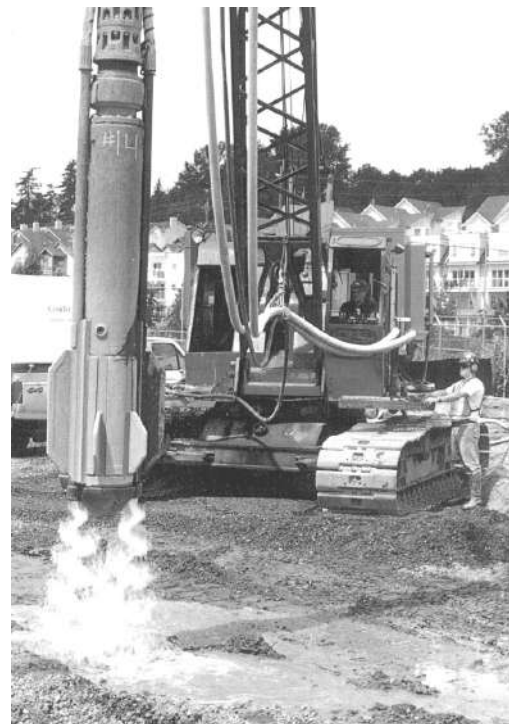
Fig. 3. Poker type V-23 vibrator (photo taken just before insertion at the stone-column location with water jets started).
