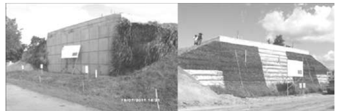
Figure 5. Photograph showing vertical face and sloping face showing metallic and polymeric reinforcements respectively.
